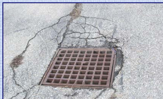
Extra attention should be given to changes and weathering in parking lot structures.
